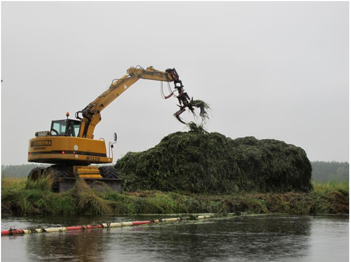
Figure 2: Staff of the local water management association removing mowed aquatic macrophytes from the river Spree, Brandenburg (photo: Jan Köhler).
