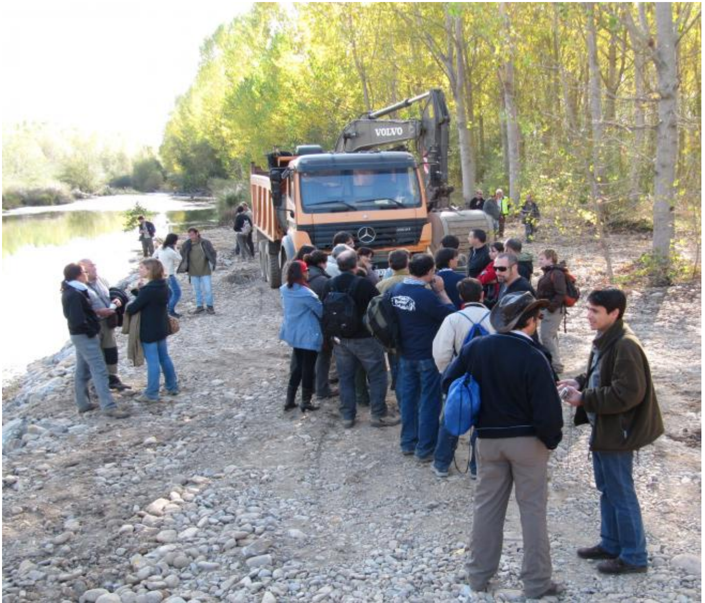
River restoration construction works in the project “Improvement of the ecological state of the Órbigo river” by the Water Commission of the Duero Basin Authority in the provinces of Leon and Zamora in north-western Spain. Photo: Bart Fokkens
